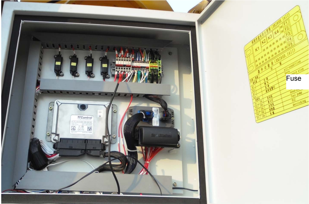
Fig. 4-7 Electrical control box wire harness
